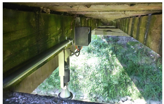
Figure 3: A gauge radar is mounted underneath a pedestrian bridge.
